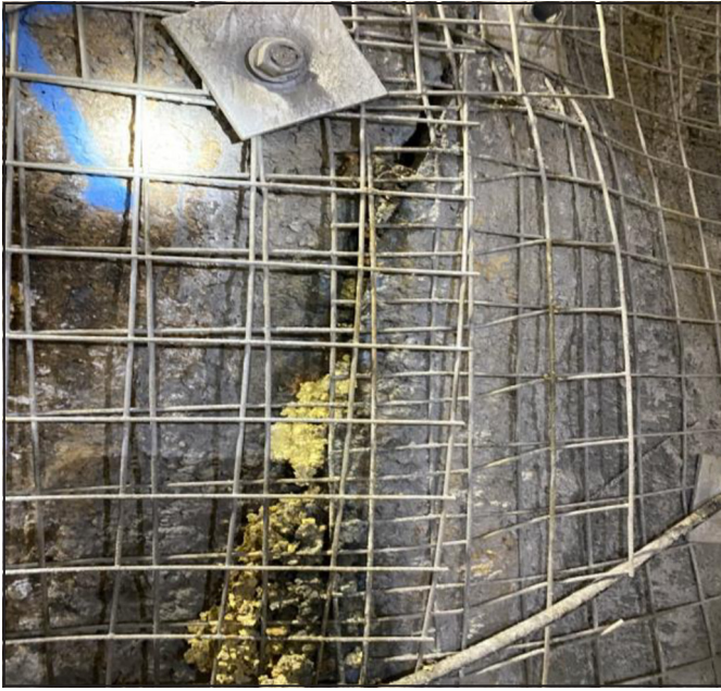
Figure 4: Examples of corrosion precipitates in cracks through shotcrete
