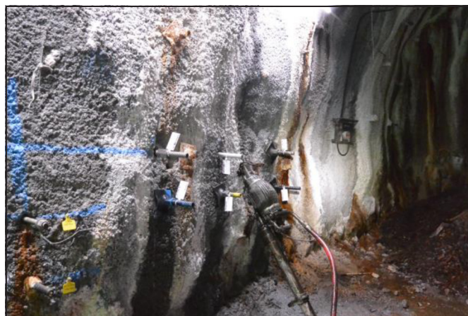
Figure 15. Various type bolts and coatings for future corrosion overcoring and testing, Old Electrical Room, 68L
