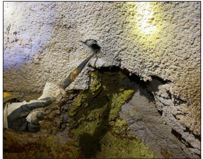
Figure 6; Corroded rock bolt extracted from 68 Level . Note corrosion although portion of the bolt was surrounded by shotcrete. Yellow (white to greenish) efflorescent minerals are recent/current precipitates
