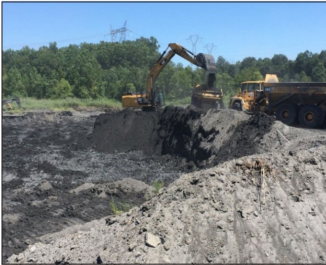
Figure 3. Dewatered ash supporting equipment
