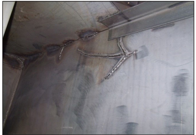
Figure 1. Typical fatigue cracking repair
