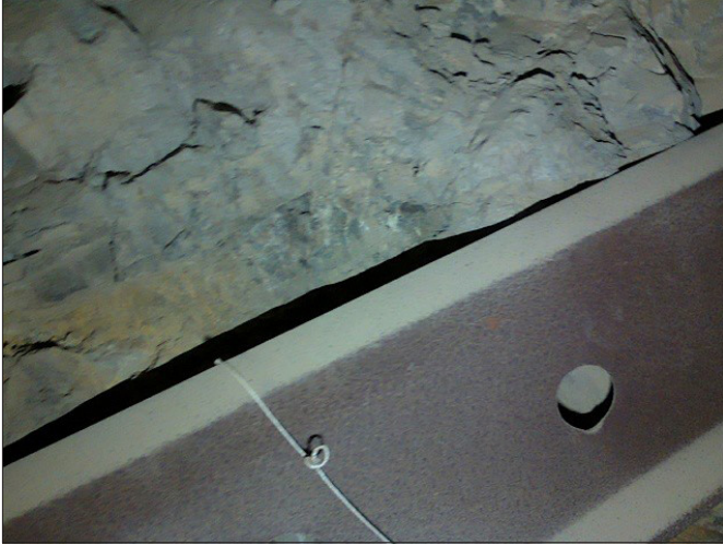
Figure 1. Shows an image of the roof with a bolted support strap, taken at the Edgar Mine in Idaho Springs, CO
