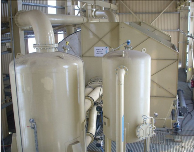
Figure 9. View of installed Bovac Disc Filter with 176 m 2 filtration area
