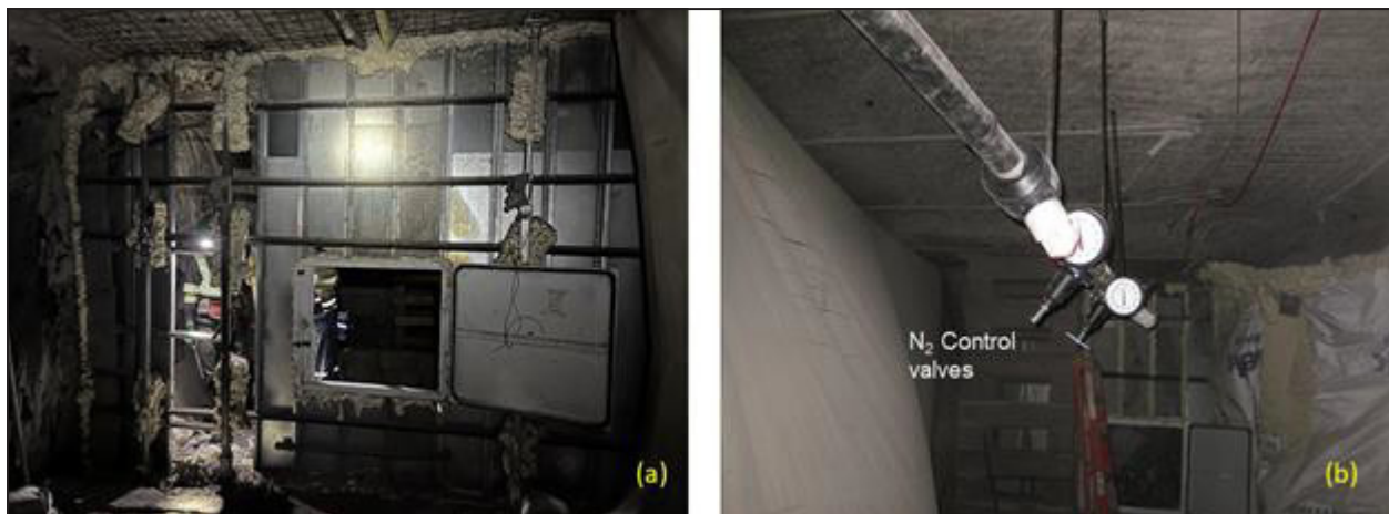
Figure 2. First pressure chamber details. (a) Kennedy stopping with personal doors to open outwards, and (b) Nitrogen injection pipeline and flow control valves
