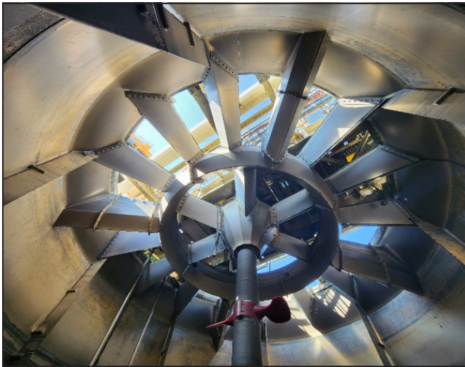
Figure 5. Internal view of Spider Crowder Upgrade in cell 7 of Line 1
