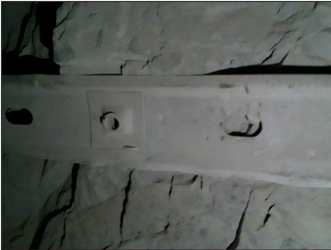
Figure 1. Shows a typical color image of the roof with a bolted strap, taken at the Edgar Mine in Idaho Springs, CO. It is imperative for any computer vision system to be able to differentiate between the strap and the underlying rock
