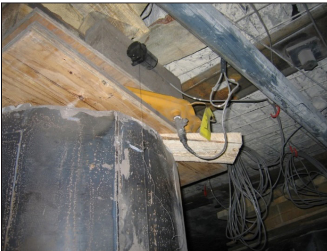
Figure 3. Complete extensometer installed on a can-type support in conjunction with a standing support load cell
