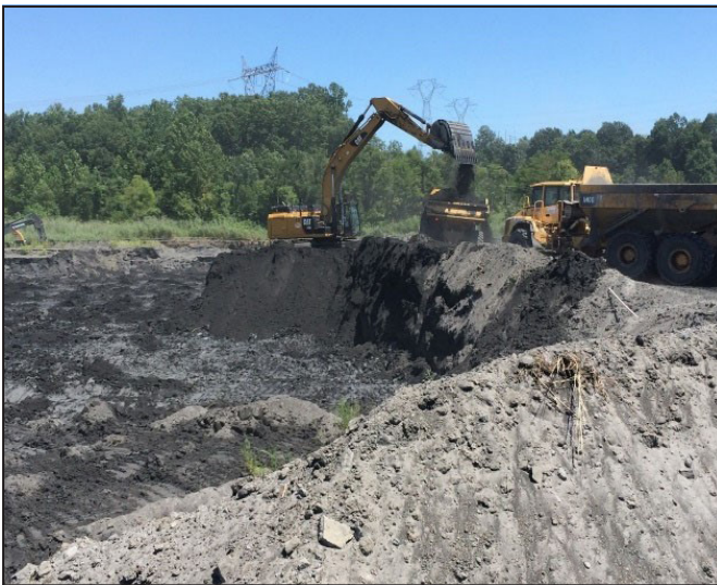
Figure 3. Dewatered ash supporting equipment
