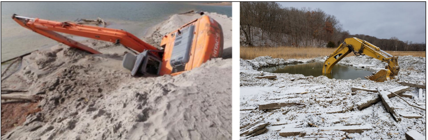
Figure 4. Equipment engulfment as a result of vibration-induced liquefaction
