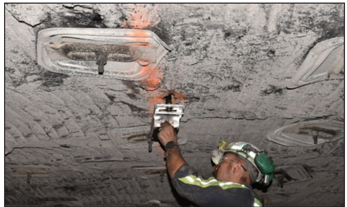
Figure 10. Photo of a researcher completing the installation of a roof extensometer using epoxy and wooden wedges.
