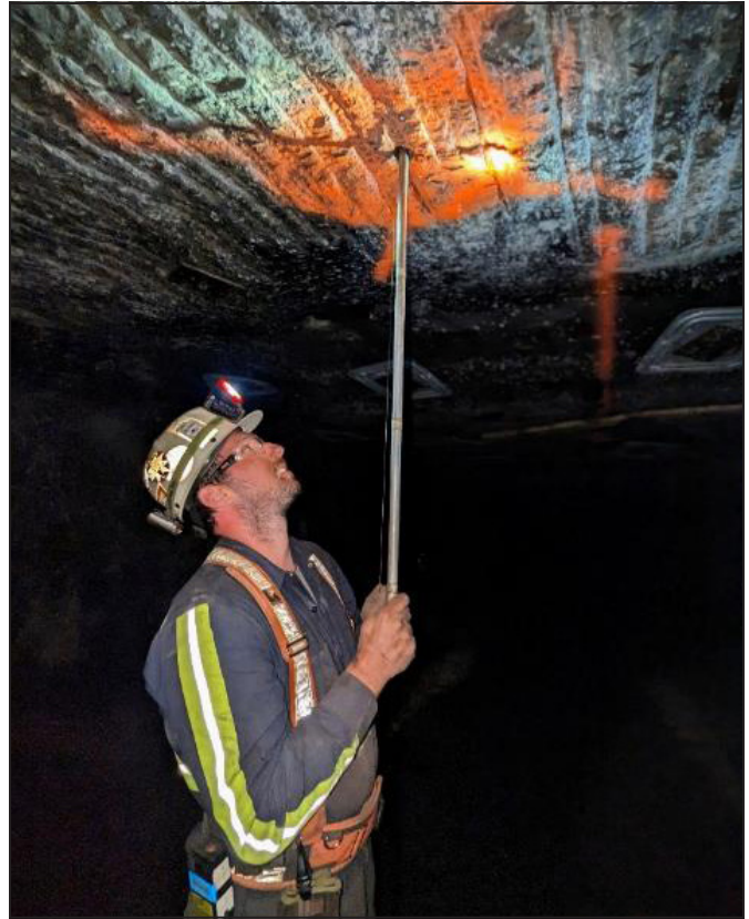
Figure 9. Photo of a researcher beginning the process of installing anchors for a roof extensometer
