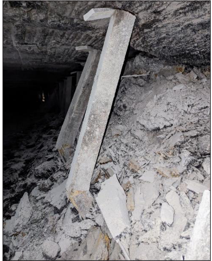
Figure 1. Example of potential rib hazards including rib sloughage and damaged supports
