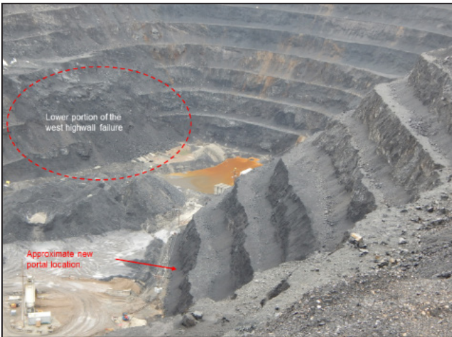
Figure 6. A view looking parallel to the highwall and catch benches above the proposed portal location
